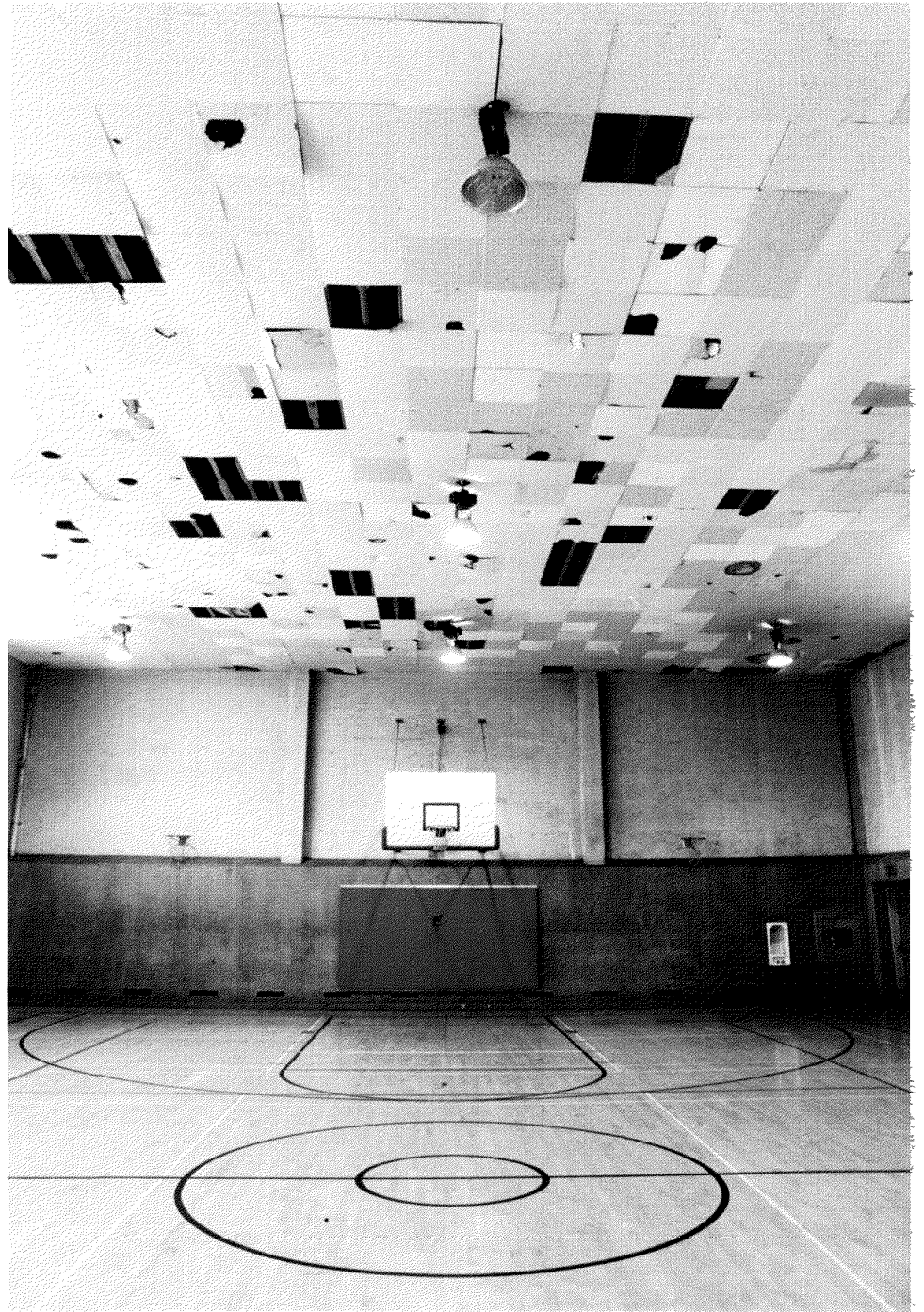
The dilapidated gym ceiling at Mark Keppel High School in San Pablo. Photo: Courtesy of the ACLU
