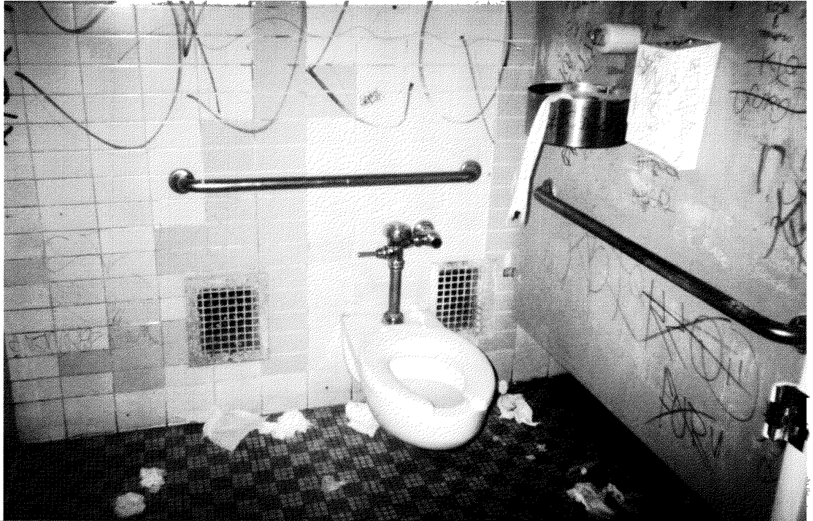
A graffiti-covered bathroom at Jefferson High School, L.A. Photo: Courtesy of the American Civil Liberties Union
